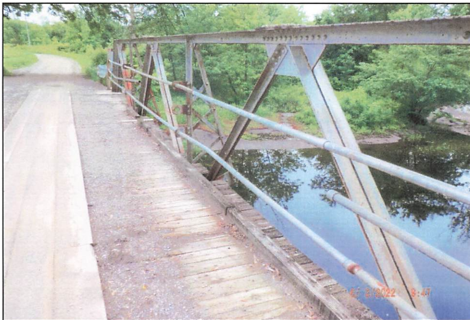
Photo 2: South Tuss and Barrier with Missing Tube Railing
