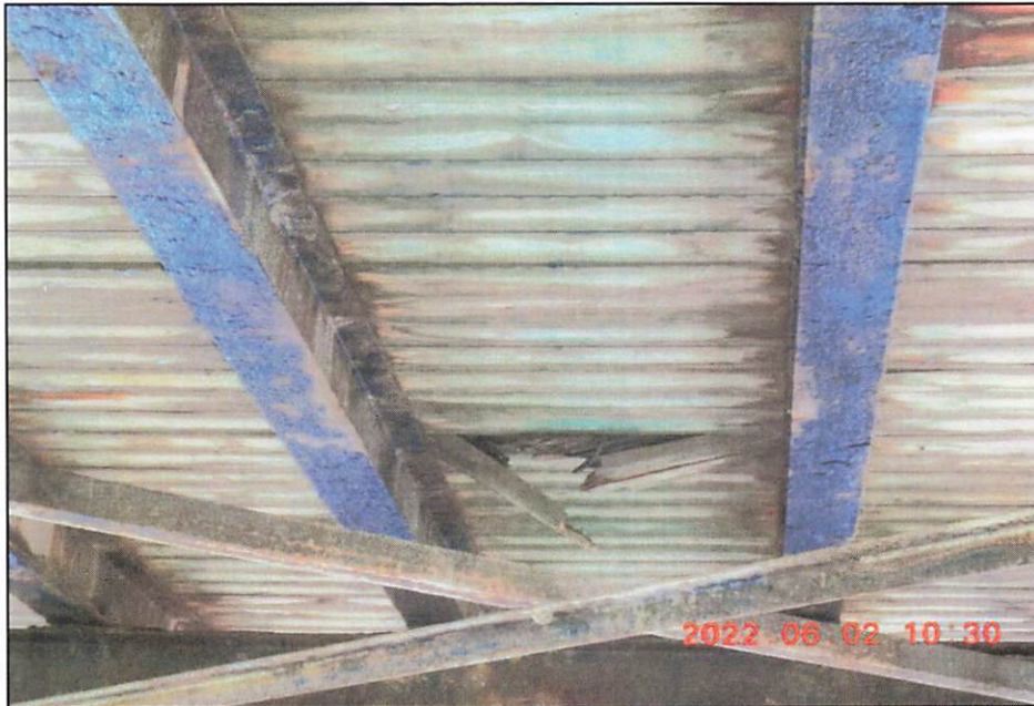
Photo 9: Localized Deck Failure
