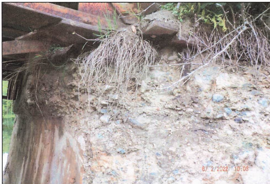
Photo 6: Loss of Truss Bearing at Southeast Abutment Wall
